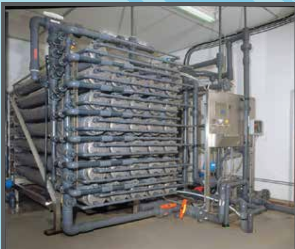
150 Cubic Meter / Day Fyne Process System in Atlantic Canada
